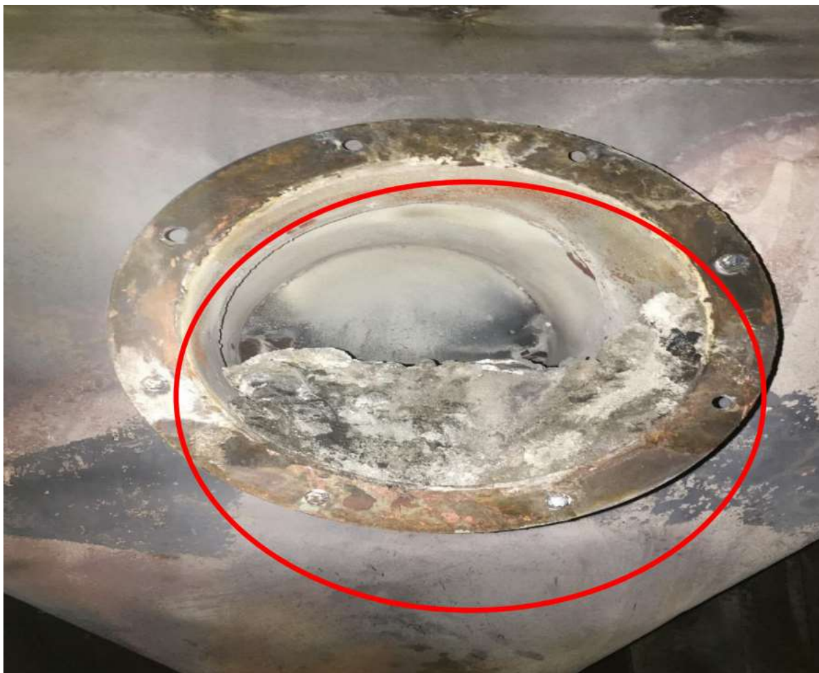
因拋光研磨機研磨鋁製品產生火花蓄熱引燃火災
