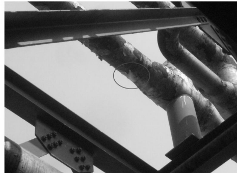
Fig. 2. Leakage point of the LPG pipeline at 9:42.
